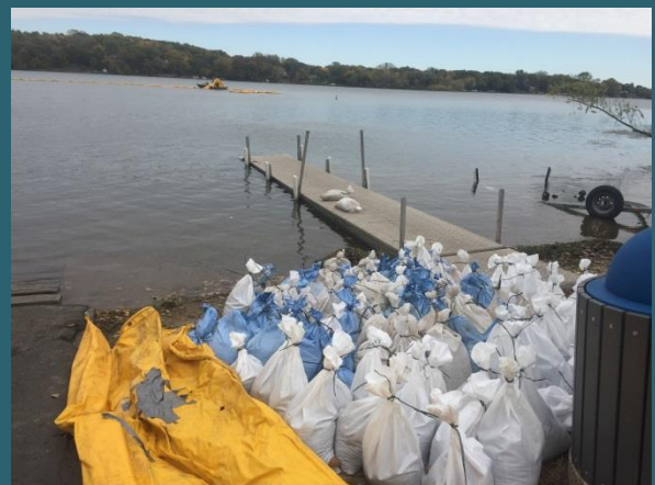
Sand bags are staged for installation of a containment barrier for the EarthTec QZ zebra mussel treatment
