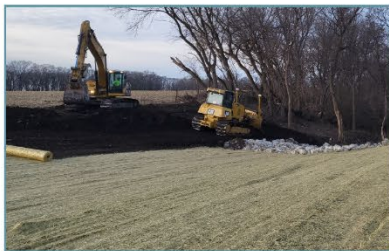
Construction of a grassed and rock-lined waterway to reduce erosion in areas of concentrated surface water runoff
