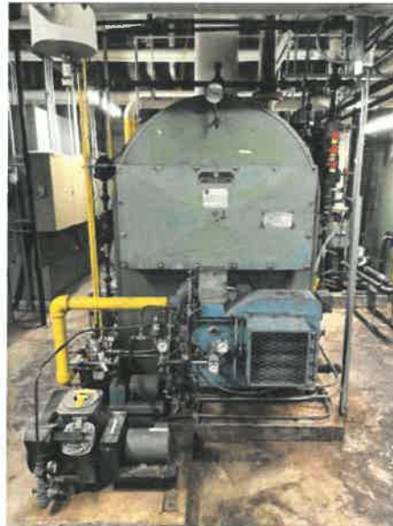
Image 1 – Image of Existing Boiler
