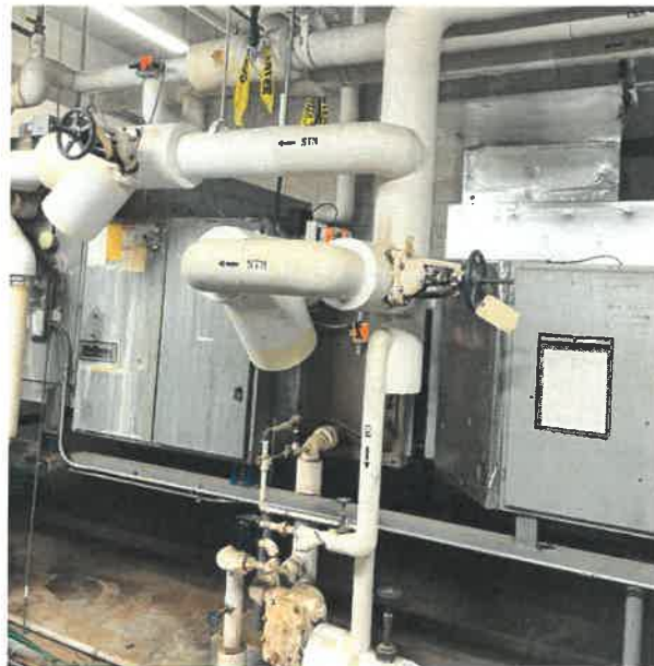
Image 3 – Existing Air Handling Unit
