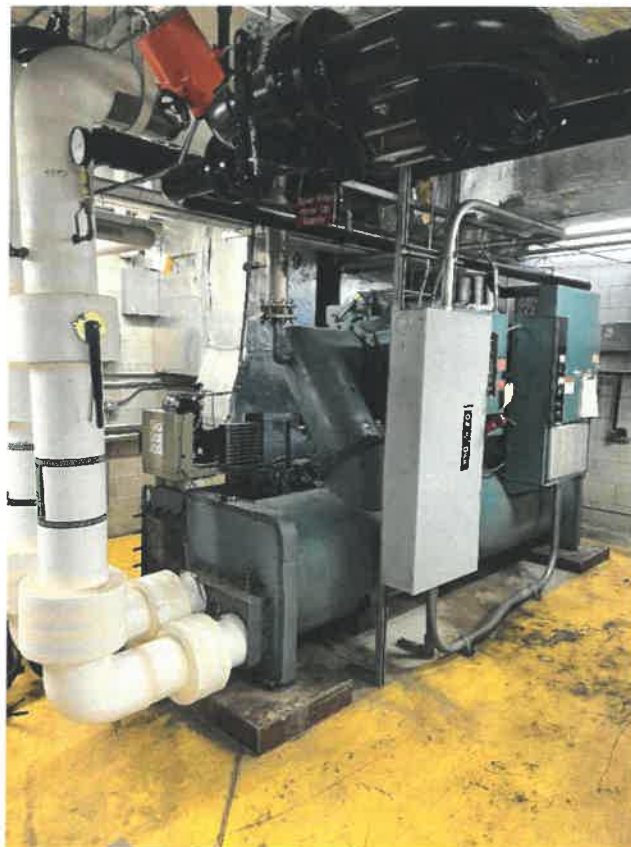
Image 2 -Existing 175-ton chiller
