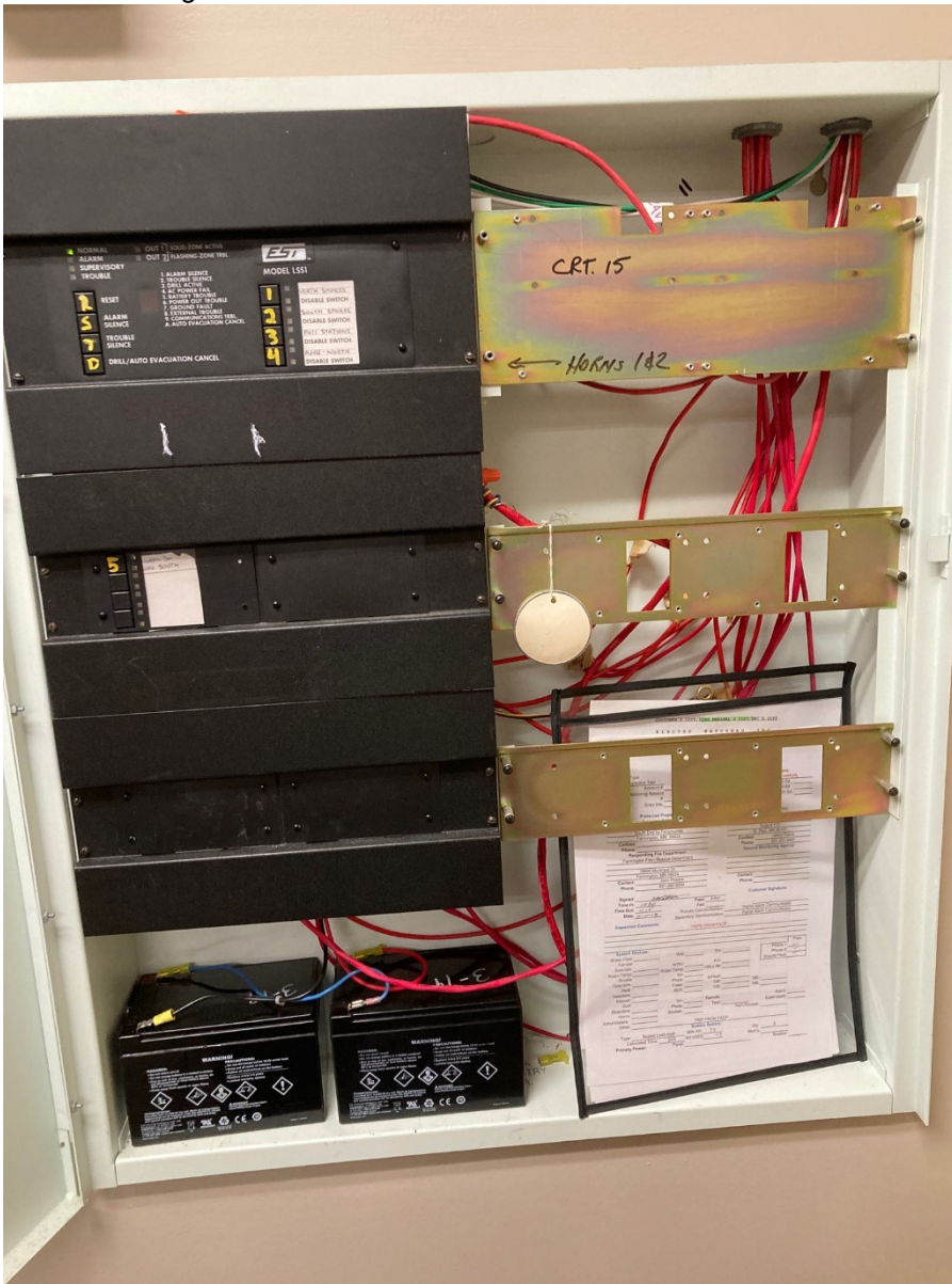
Figure 1 - Picture of the Current Fire Panel
