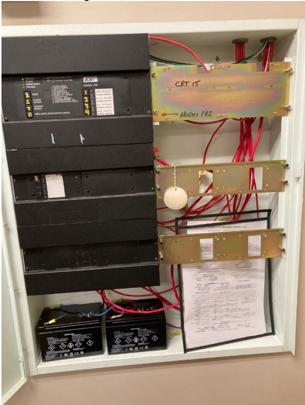
Figure 1 - Picture of the Current Fire Panel
