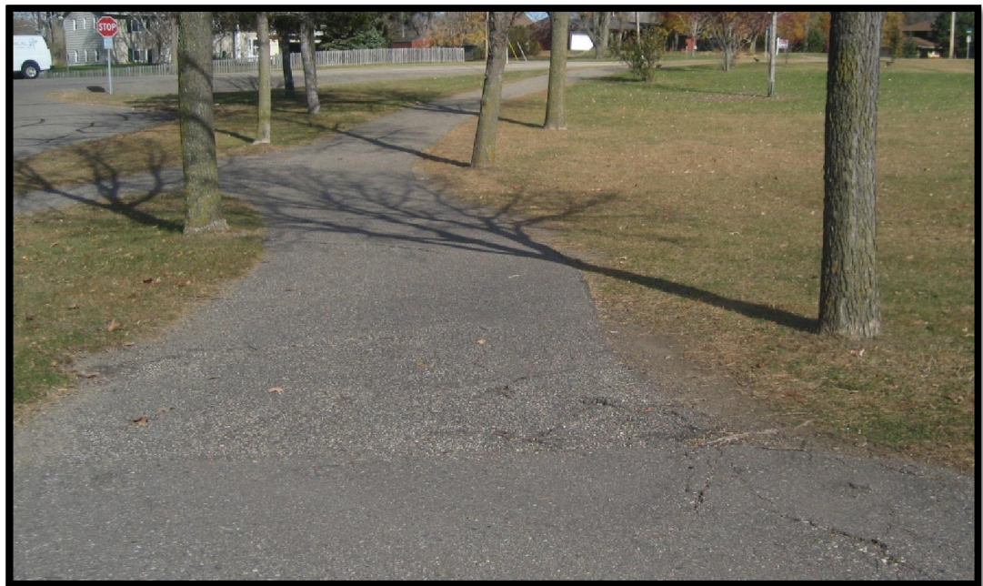
Existing trail condition between the northeast corner of Pilot Knob School and Lone Oak Road
