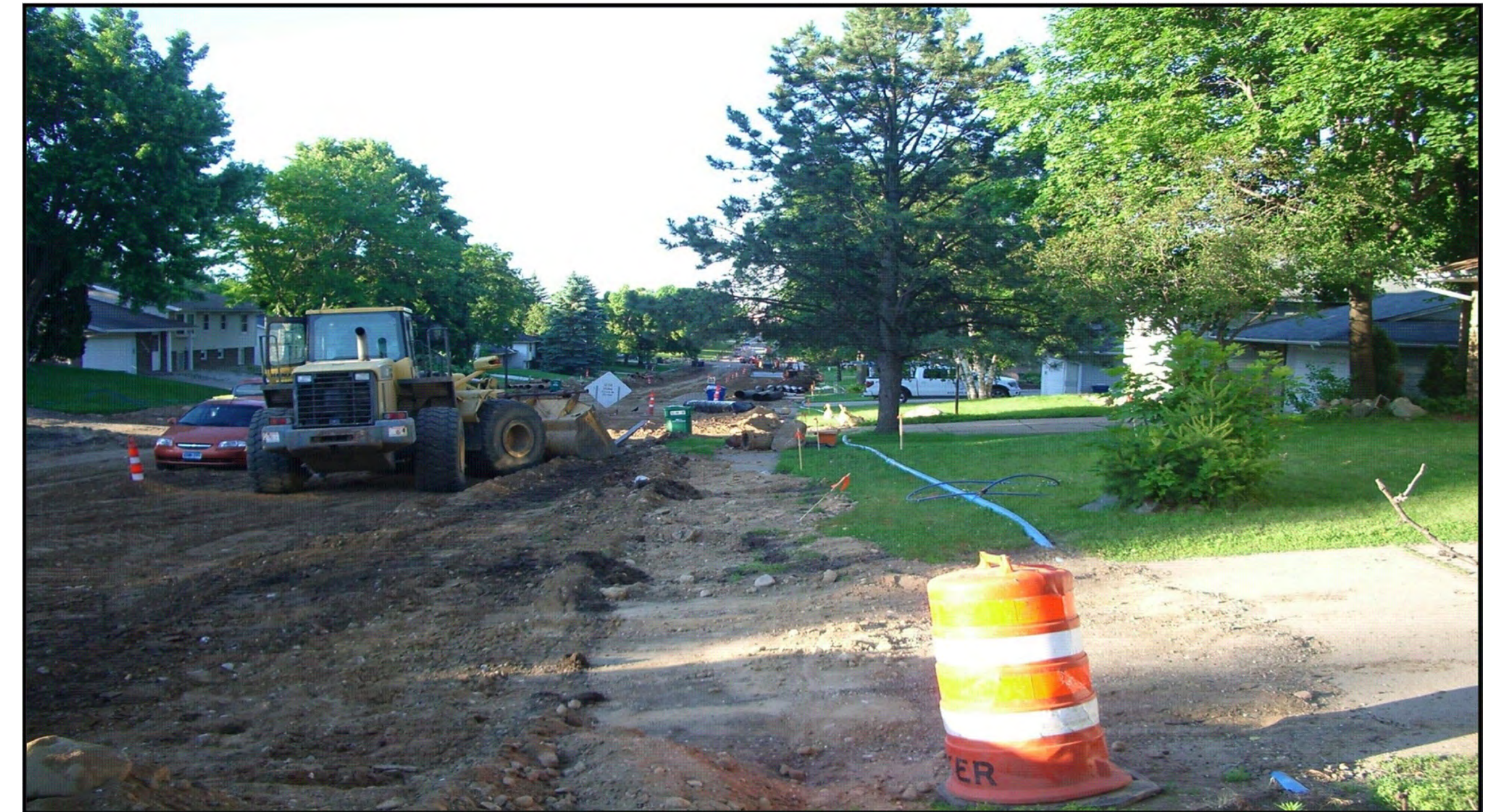
Temporary Water Service
