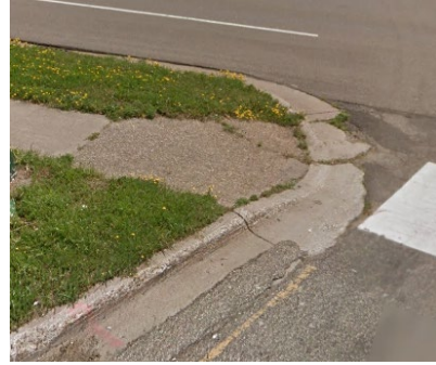
Example of a poor or non-compliant pedestrian ramp
