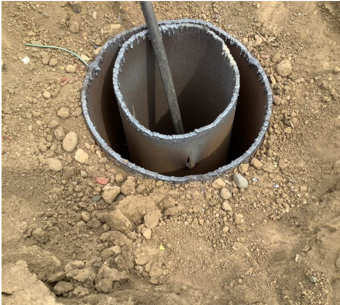
Figure 2. Open Groundwater Well
