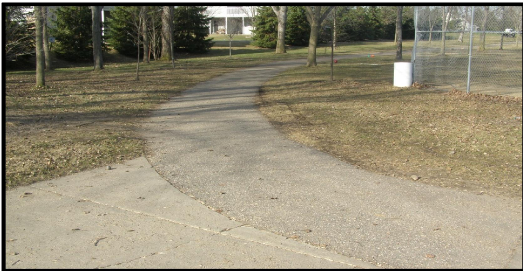
Trail connection through Newell Park to the back of Cedar Park Elementary.
