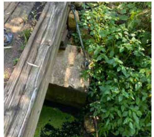
Trout Brook footbridge damage
